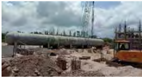
Site erection of 4.5m dia x 50m long (6 nos.) air Storage Vessel
